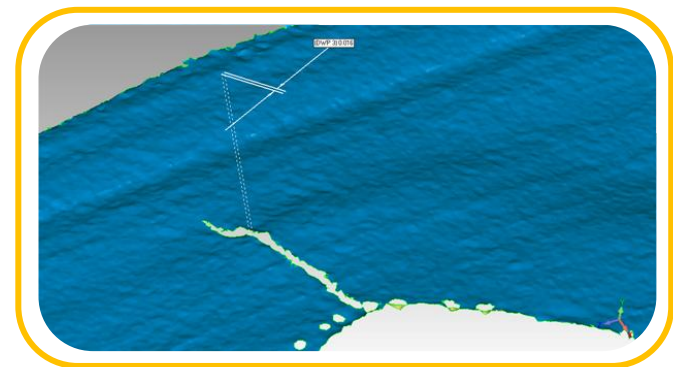
CAD model of a BWR steam dryer door indicating both precise crack length, width and surface condition.
